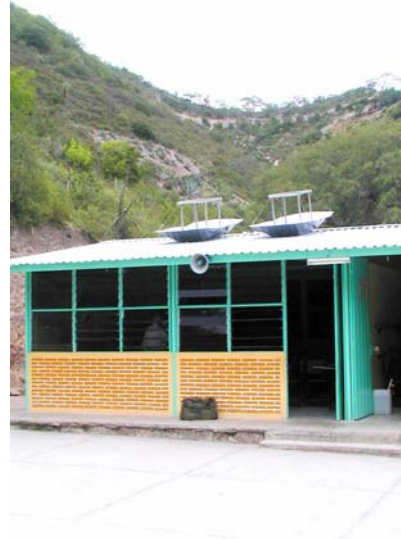
Fig. 7. Two bifacial solar panels with reflectors on the roof of rural school
